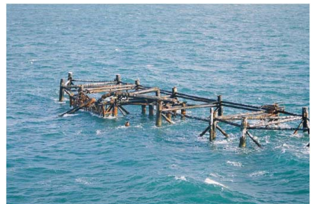
Figure 4.4 Destroyed Platform in the South Timbalier Region
