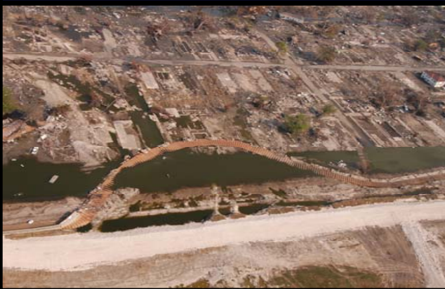
Sheetpile Floodwall Collapse
