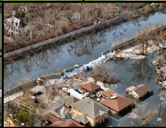
Canal Breach at Mirabeau
