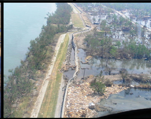
Failed Floodwall at Triumph
